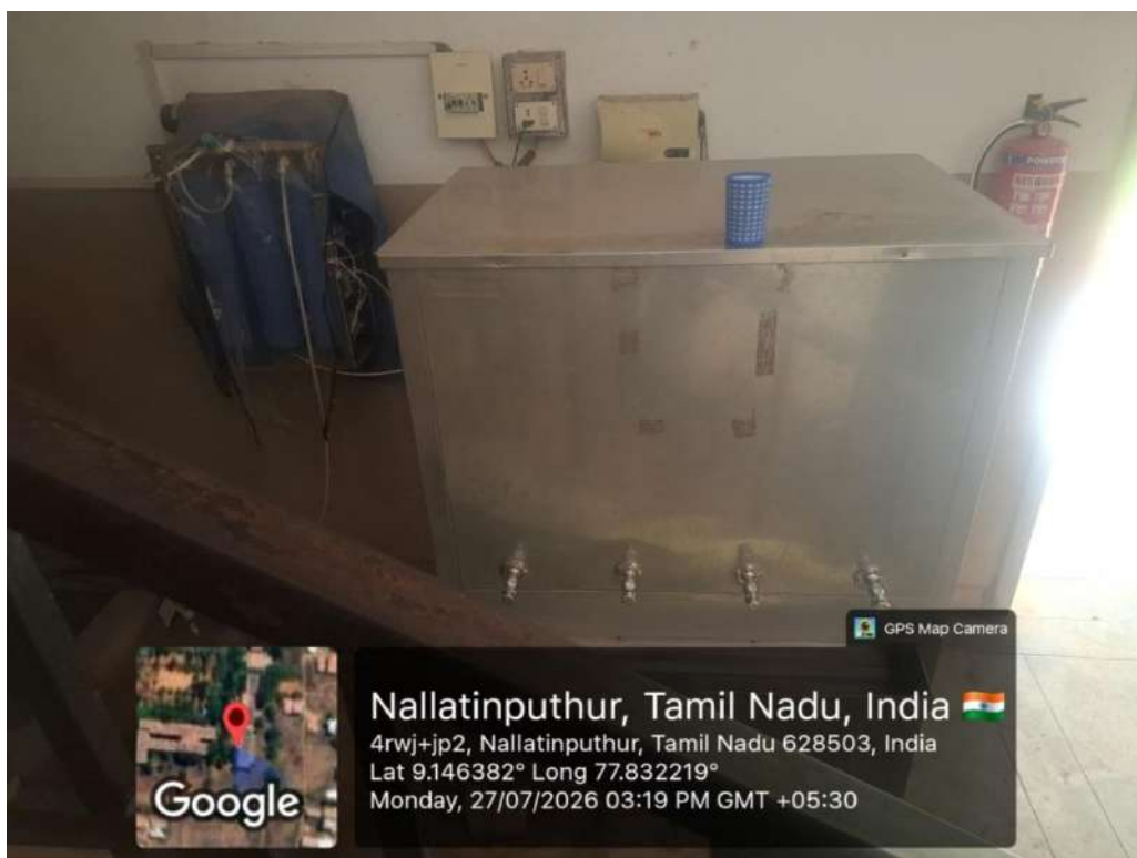
RO water purification unit installed in the CSE Department
