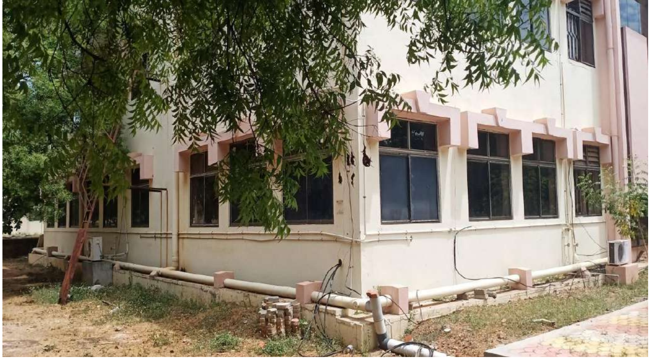
Rainwater Collection Pipeline from Rooftop to Harvesting Pit, First Year Block
