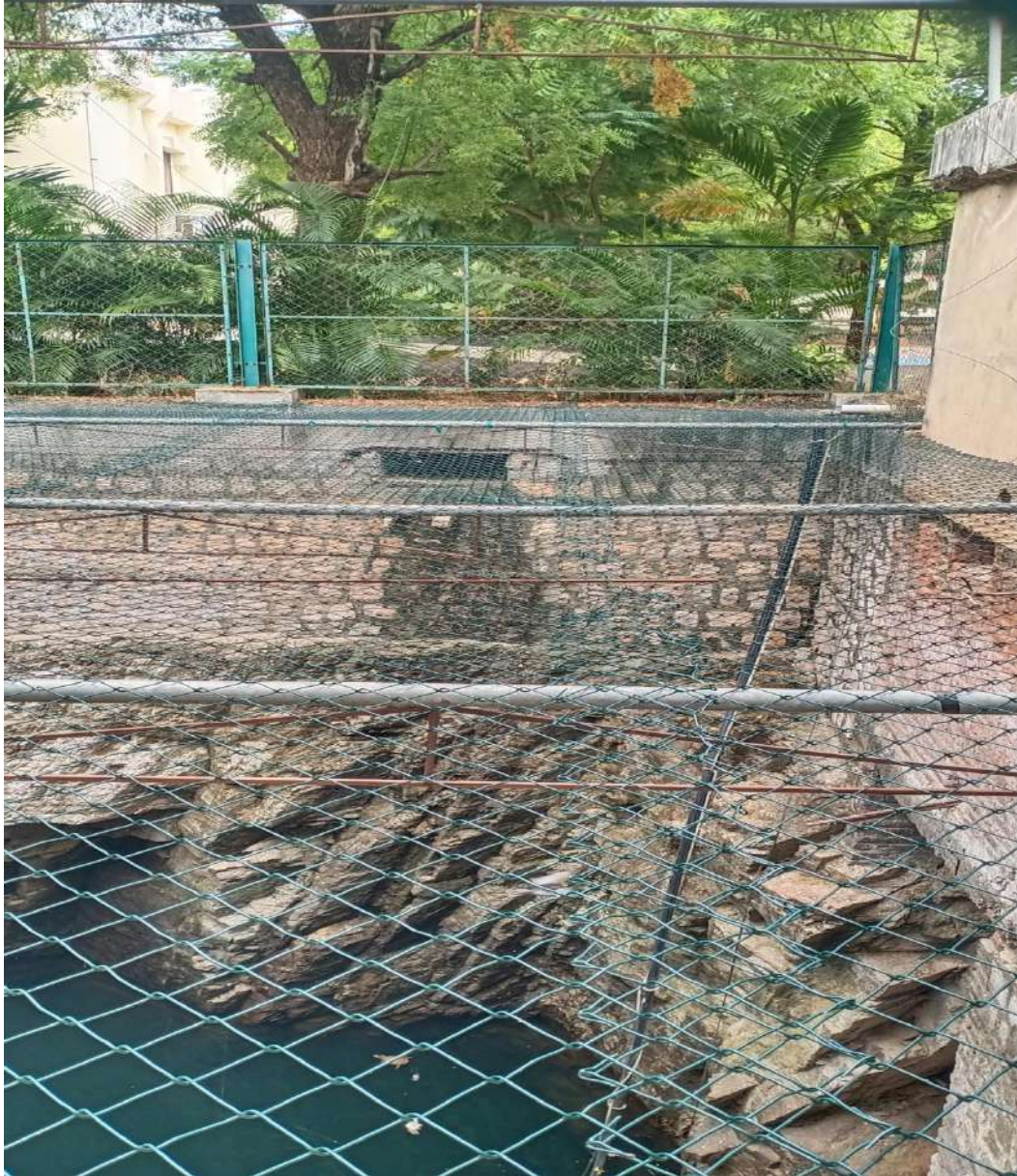
Rainwater Harvesting Pit, Secured with Protective Fencing, Opposite to Admin Block
